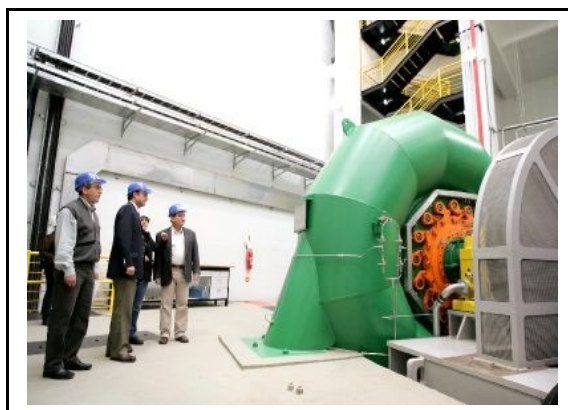
PCH Esmeralda-RS com 22 MW
